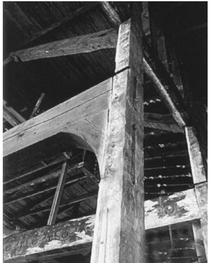
Figure 2 The Daniel Pieter and Jannetje (DeForest) Winne house, c.1750, stripped to its frame. Photograph March 2003.
